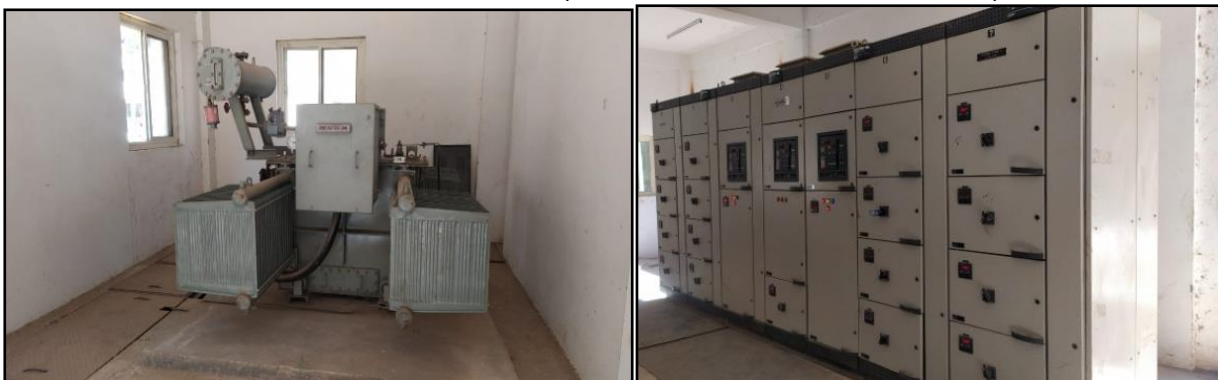
Indoor 11/0.415 kV (800 kVA) Transformer
