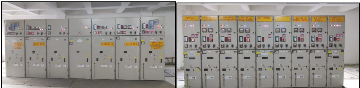
33 kV Indoor panel
