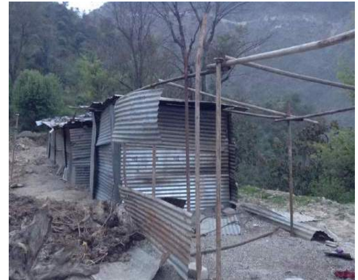
Figure 2. Tin structure destroyed by wind.
