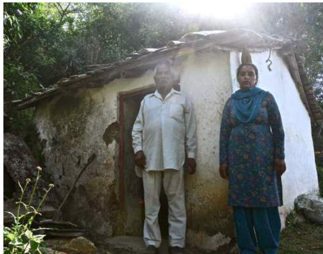
Figure 12. Gharat in disrepair in Manyana,
